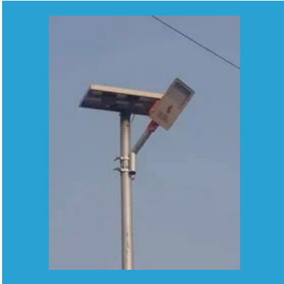
Steel Street Light Pole
