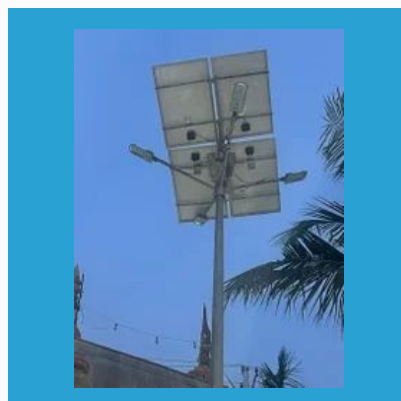
Solar High Mast Light
